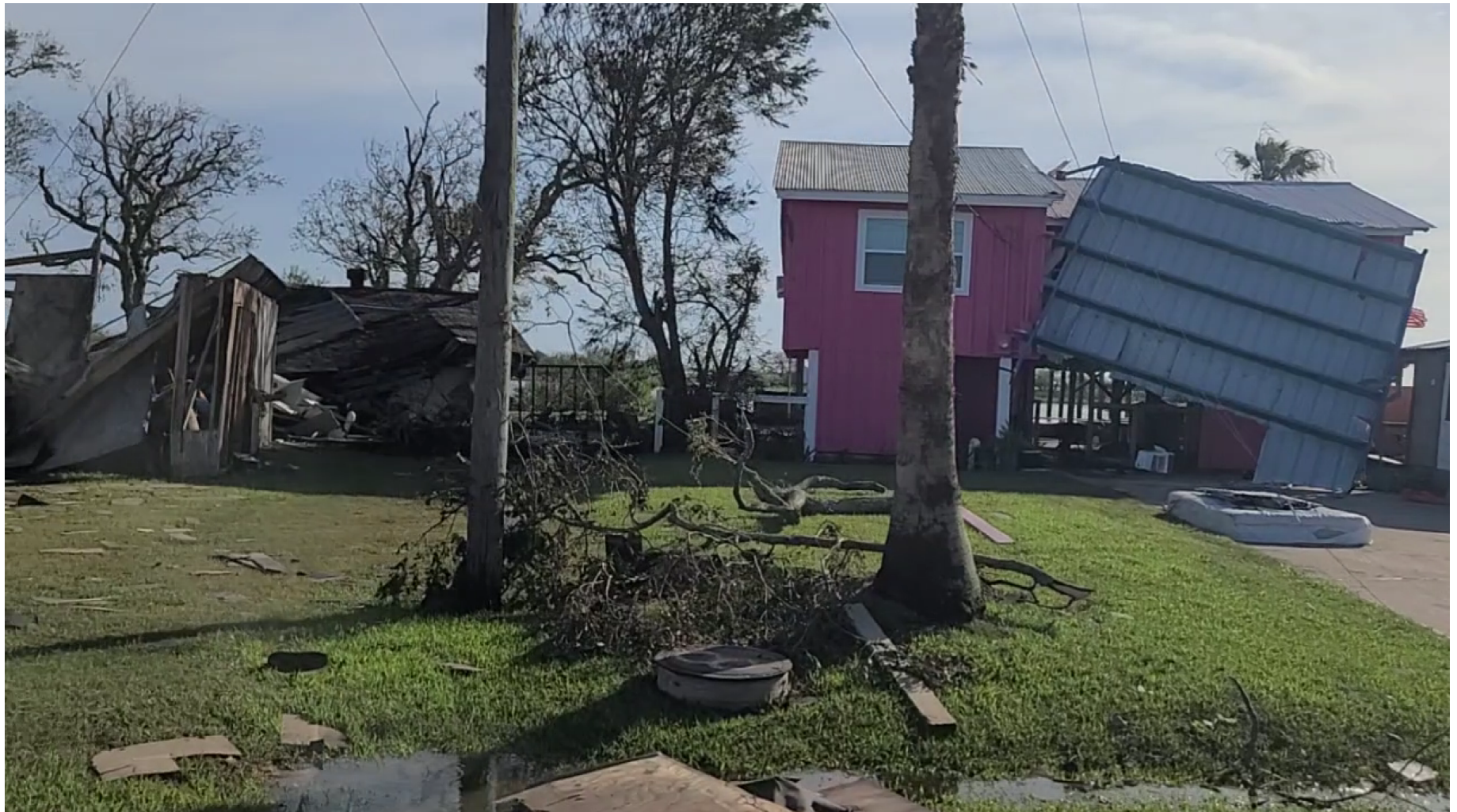
Figure 12. Wind and storm surge damage to homes and trees at Sargent, Texas, caused by Hurricane Beryl. Image courtesy of Josh Morgerman/iCyclone.
